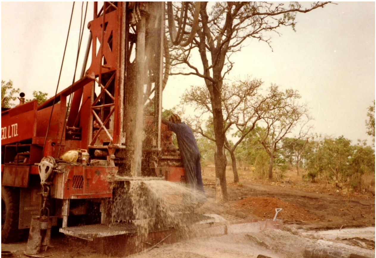
FIG. 6-05 Kwara State of Nigeria, 1985 WATER, WATER !
