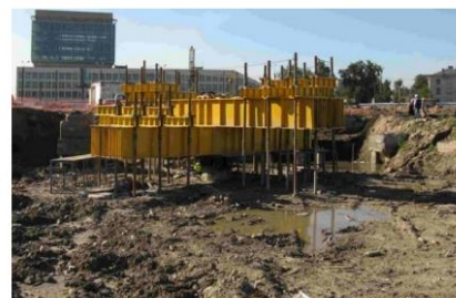
Figure 3. 30 MN top down reaction beams on a barrette test with multiple anchor piles (Fugro).
