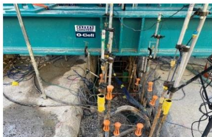
Figure 2. Bi-directional loading test on a pile with concrete cut-off level 12.3 m below ground level (Fugro).
