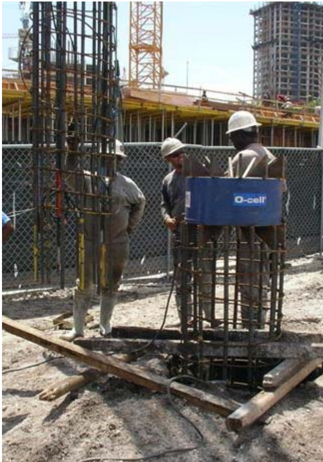
Figure 5: A 660mm O-cell about to be integrated into upper section of reinforcing cage.
